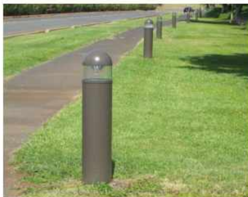
Bollard Lighting along a Trail
